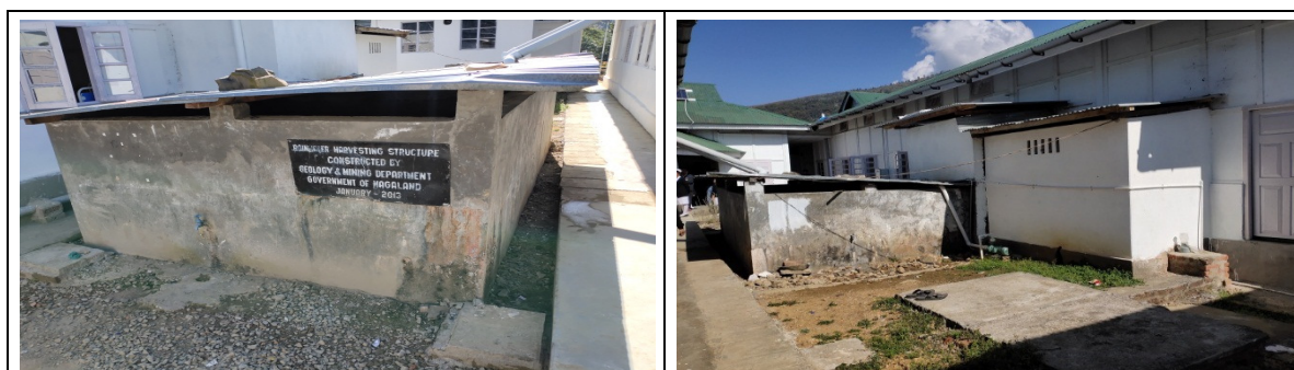
Photograph 5.18: Water storage tanks in DH Wokha
