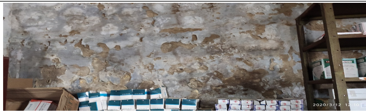
Photograph 5.6: Seepage in an entire wall of storeroom where medicines are stored in DH Kohima
